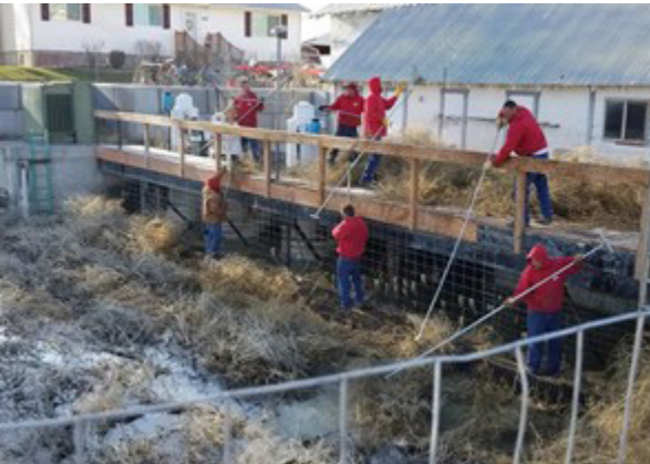
A large crew manually removes tumbleweeds from the original screening system in the Owsley canal.
