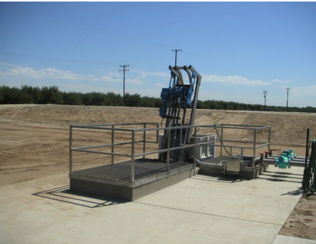
The Duperon ® FlexRake ® removes all debris damaging to the vineyard's evaporative ponds.
