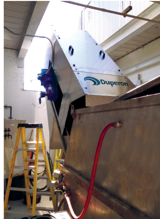
The Duperon® FlexRake® was installed using the hole in the roof that was originally created for maintenance of the previous equipment.
