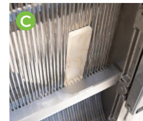
Rapid re-engagement removes large debris without shutdown to return scraper into the bar screen faster
