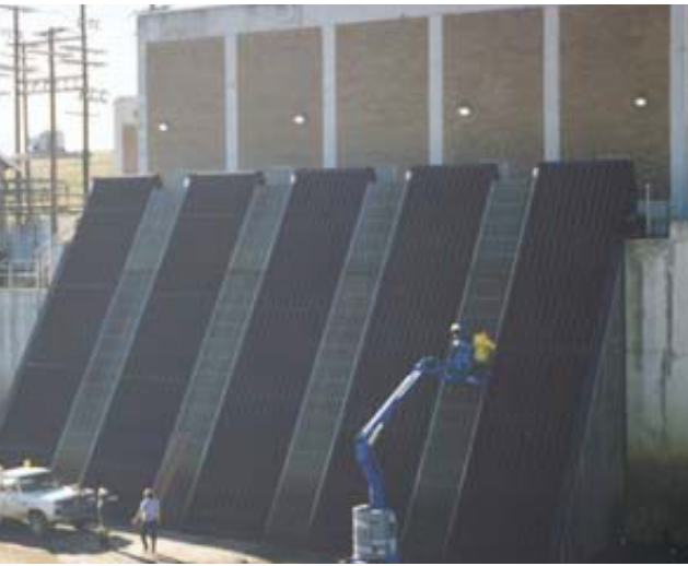
The Duperon ® SCTs at Hampton Road Pump Station, more than 100 feet long
