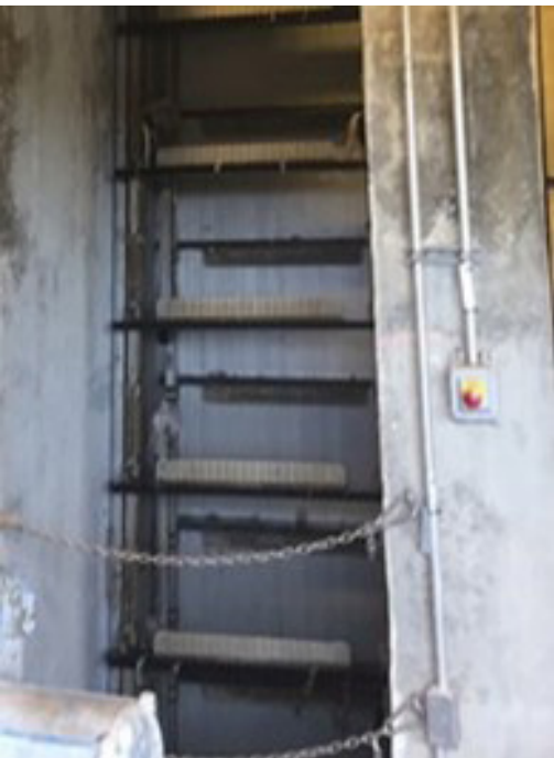
Main Pump Station intermediate level
