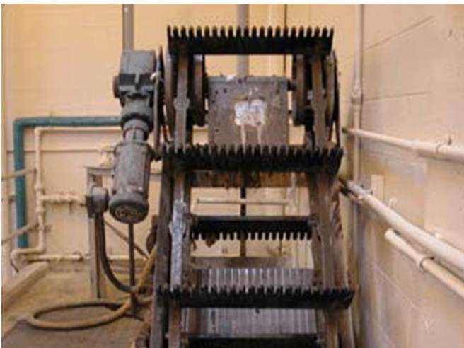
The Duperon ® FlexRake ® FP was commissioned in 1998 and has been running strong, and maintenance-free for over 20 years.
